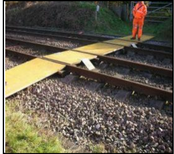
Figure 18: Crossing surface viewed from the north side of Moss Lane Farm level crossing. November 2013
